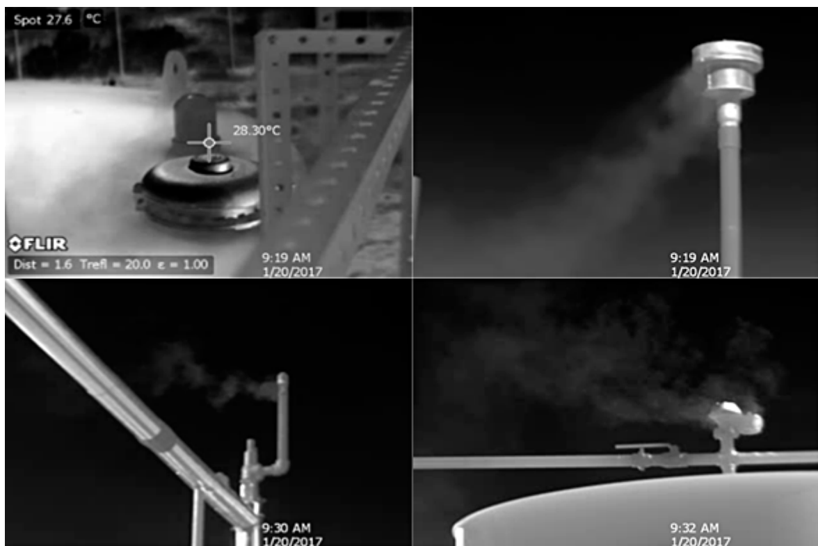
Figure 60. Emissions from closed vent systems that route emissions to a control device. Top left clockwise: tank thief hatch; spark arrester on dehydrator knockout tank; pressure relief valve on dehydrator regenerator stream; tank pressure relief valve.
