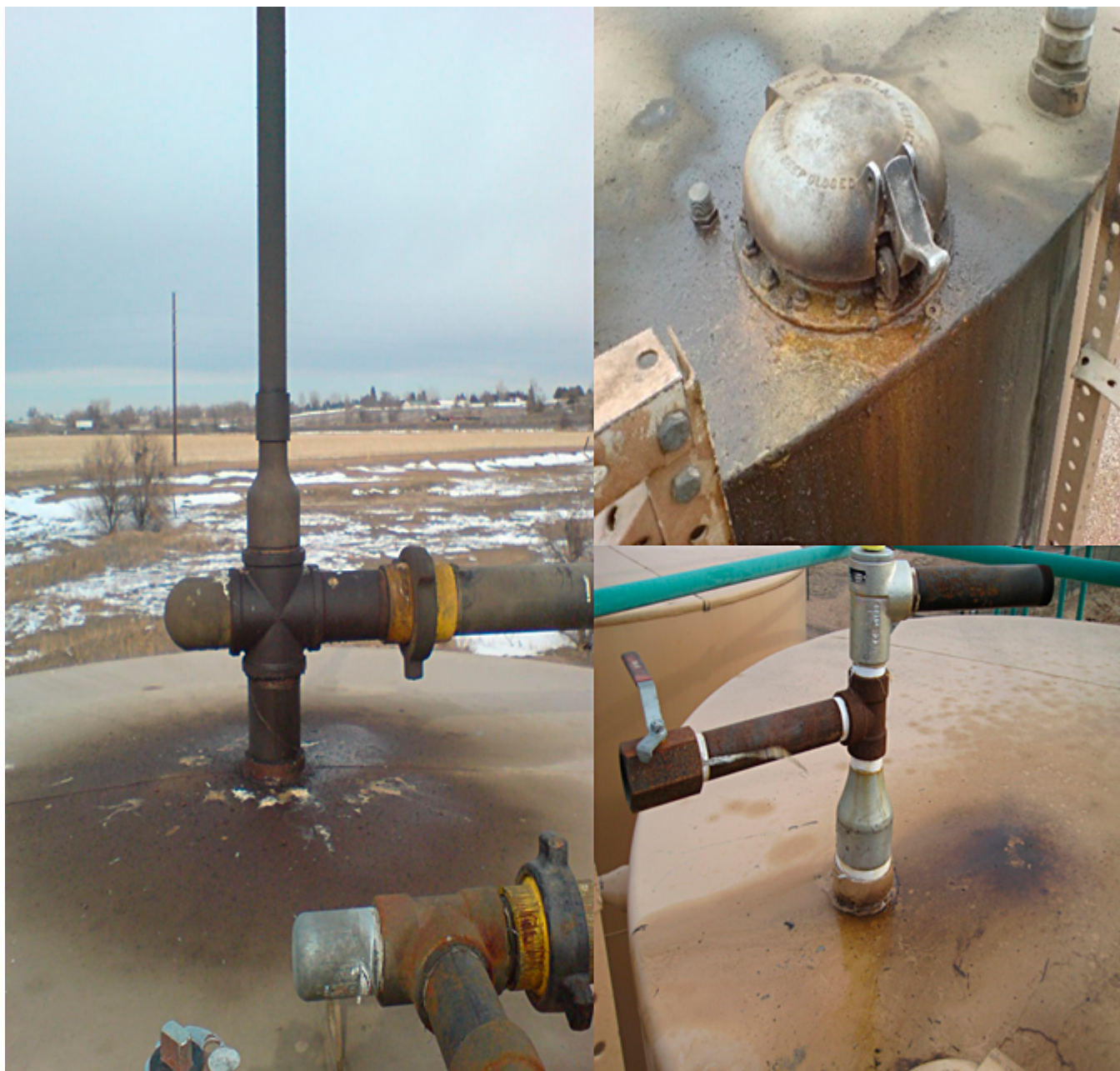
Figure 61. From visual observations, examples of “burped up” oil under and around pressure relief devices (thief hatches or valves) of controlled tanks at compressor stations, indicative of over-pressure events where gas emissions would also be present.
