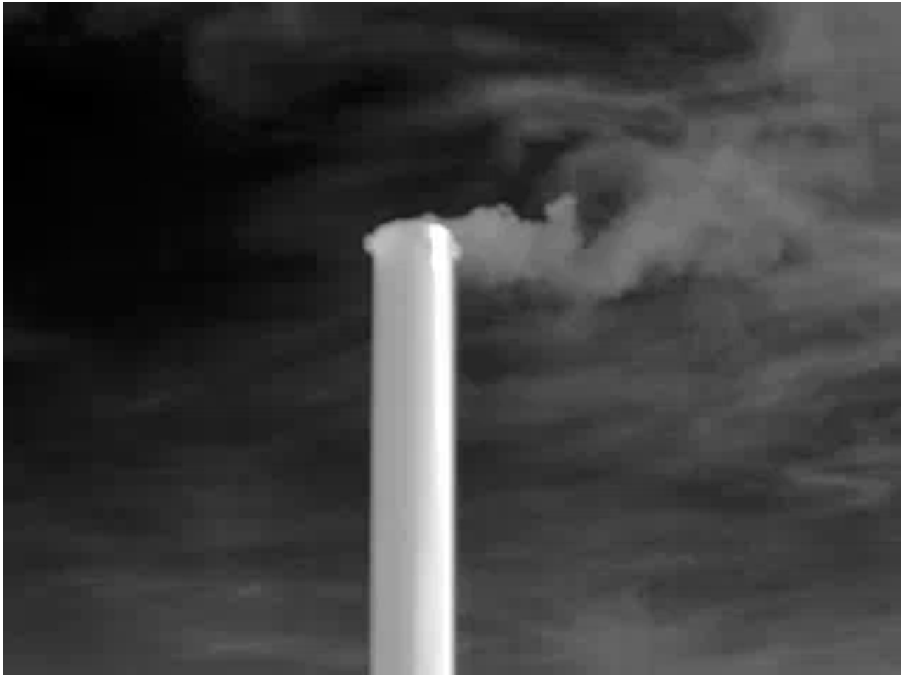
Figure 57. Centralized blowdown stack in a compressor station where several pieces of equipment are piped to.
